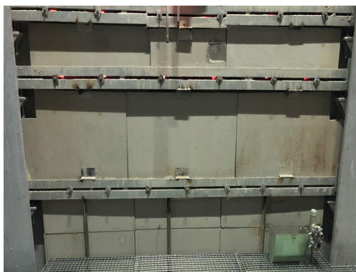
Figure 6: Completed glass regenerator refractory lining system made up of JM23 IFB and Superwool Plus Blok 800
